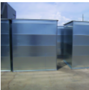
TDF - Coil Line Ductwork
